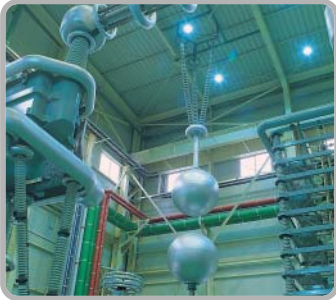
High Voltage Test / Impulse Test
